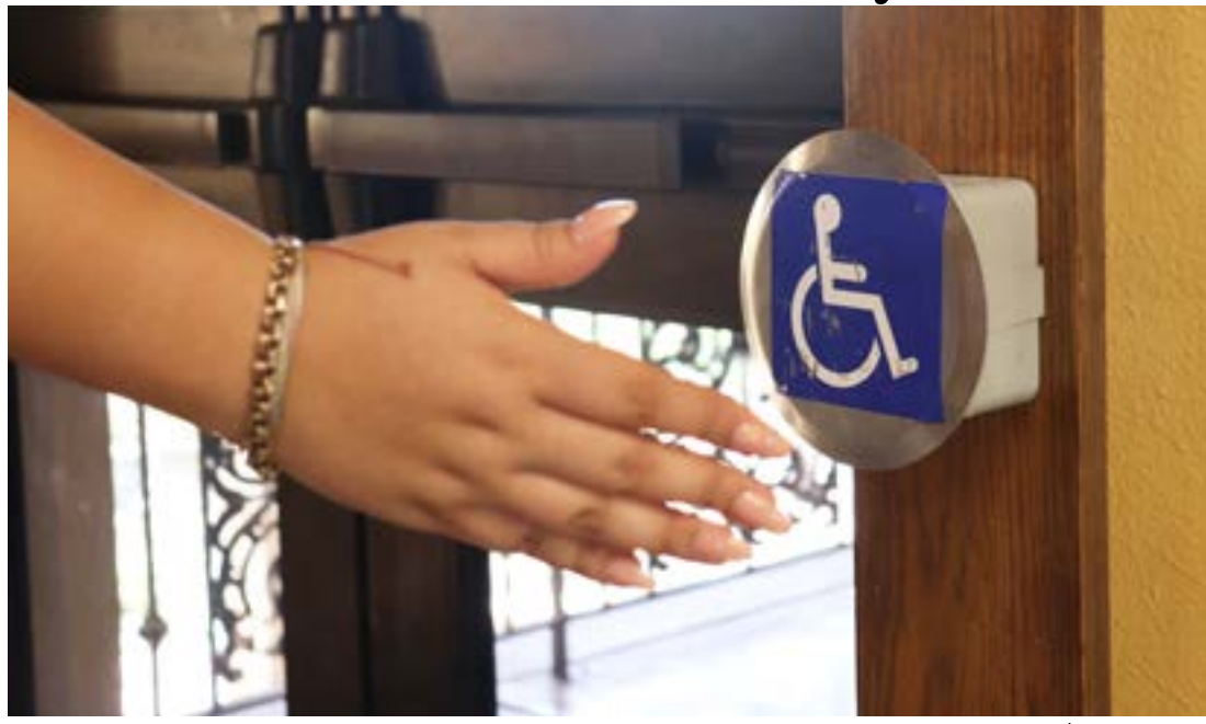
Shown is a broken automatic door button for handicap access in the Student Union on the Brownsville campus, leaving users facing accessibility challenges. The UTRGV Student Accessibility Services department is working to restore full functionality to the building entrances on all campuses.
